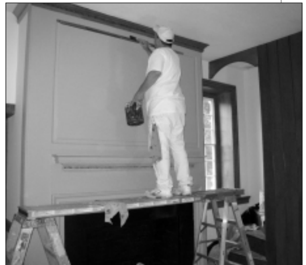
A painter applies the first coat of paint to create the verdigris finish that will found in four rooms.
